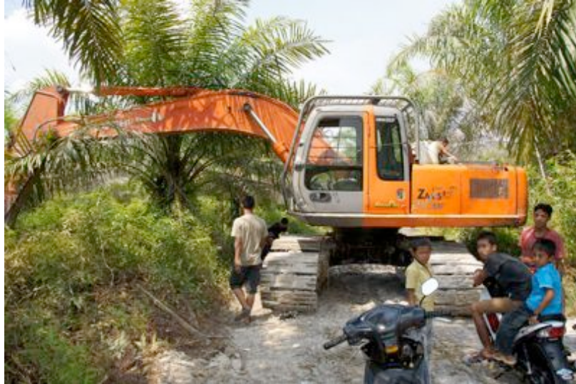
The problematic excavator once again out of order (piece of engine broken)
